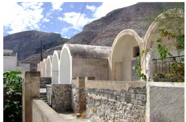
Figure 8. The actual state of the Post- earthquake housing, around sixty years after their construction.
